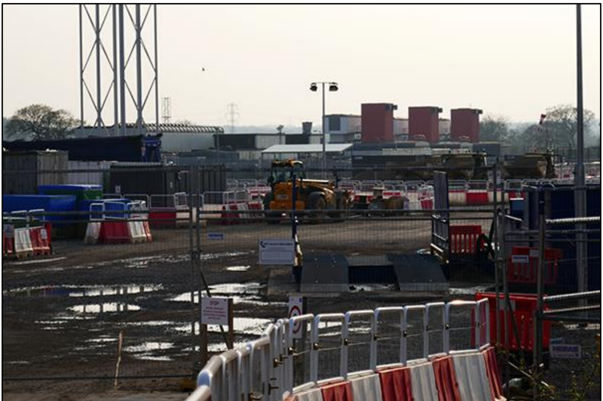
National Grid gas compressor station
